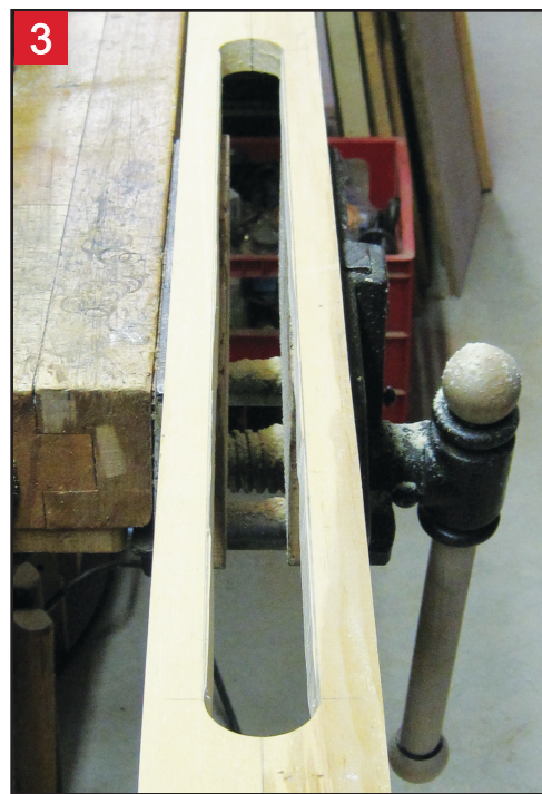
Drywall screws applying shop jig to maple bass neck, with no root-size relief holes drilled, but with no neck splitting!
